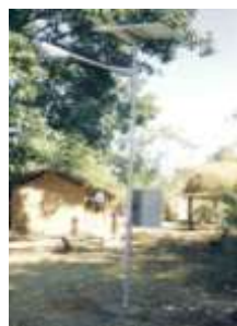
Solar street lighting
